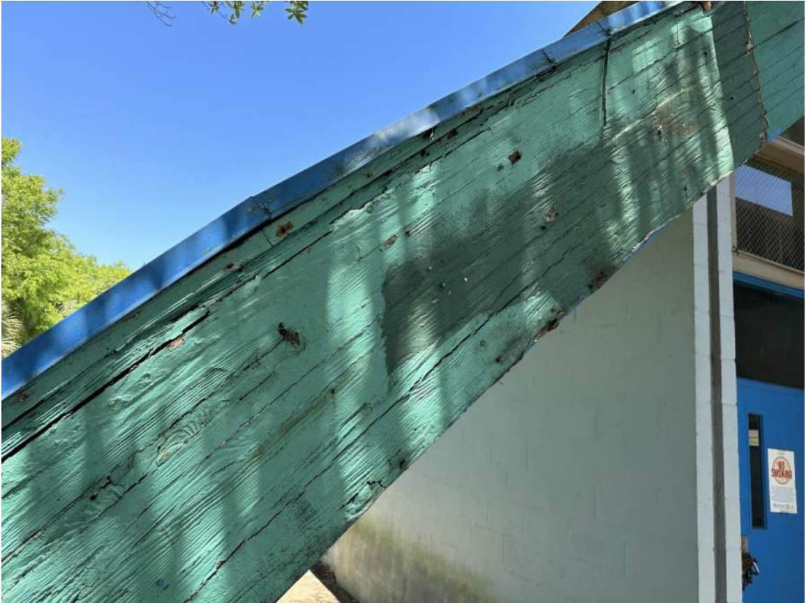
Arch #1 at South Side of Bldg (Viewing West End of Arch between Concrete Buttress and west wall) NOTE: Excessive / Severe Decay & Delamination
