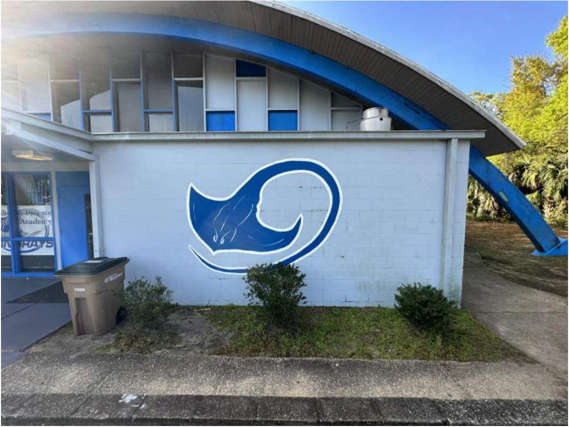
Arch #7 & Cracked CMU Wall at North Side of Bldg (Looking South)
