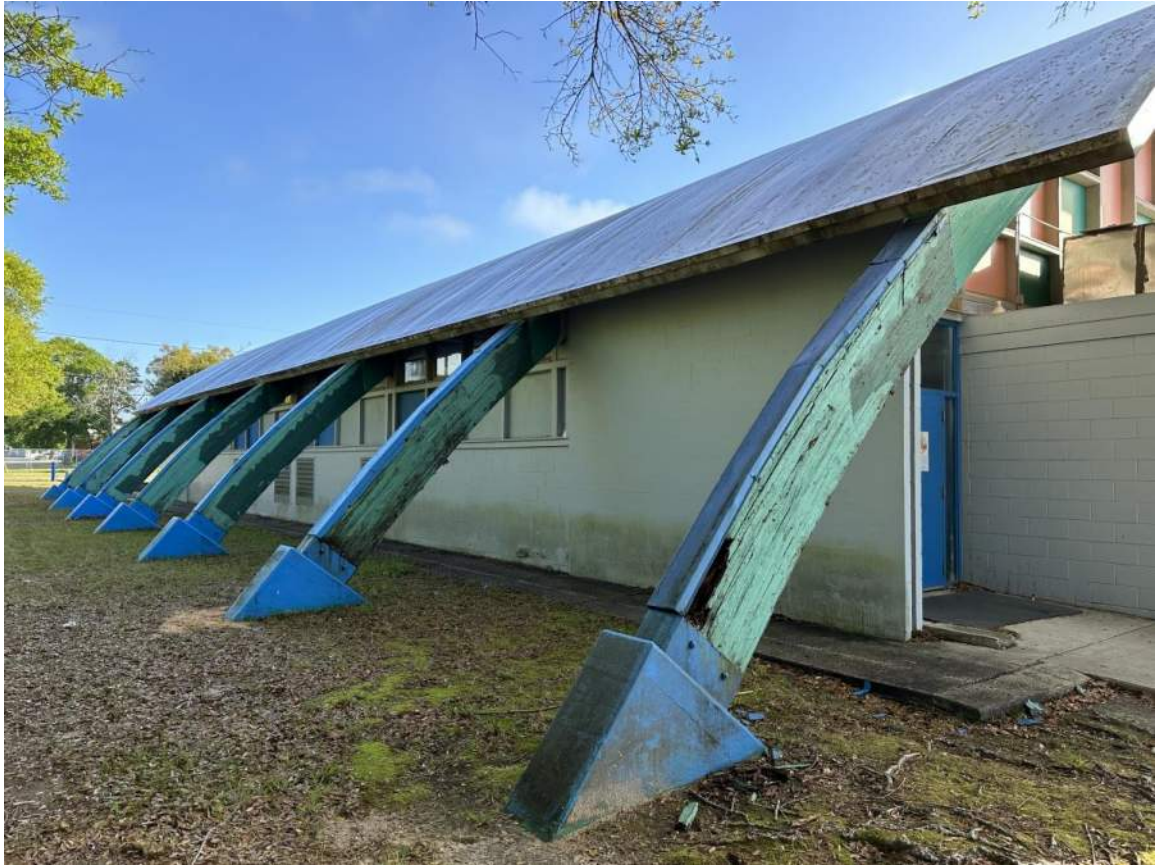
Arch #1 in foreground of photo at South Side of Bldg (Viewing West End of Arches; Looking NE)
