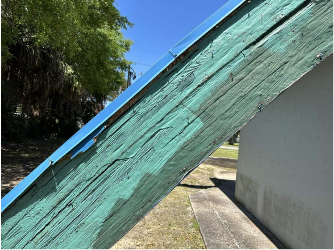
Arch #6; West End of Arch near NW corner of Bldg (Viewing West portion of Arch just above Concrete Buttress)
