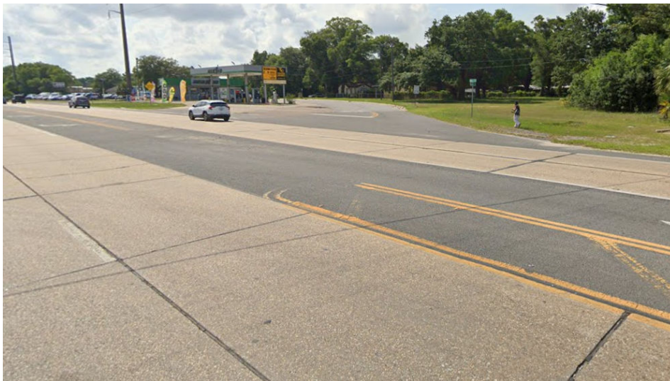
Lack of pedestrian crossings or sidewalks on W Navy Blvd (Highway 98).
