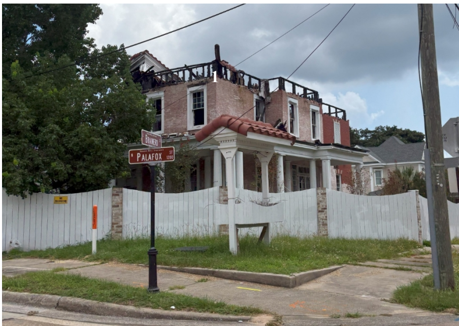
Vacant and fire damaged structure on Palafox Street.
