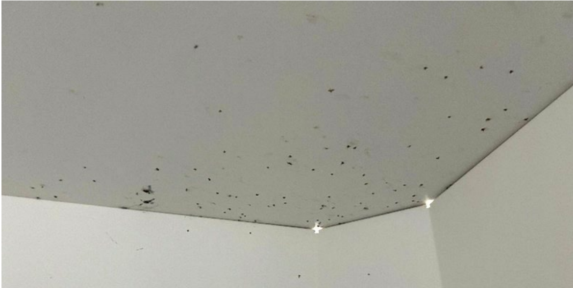
Figure 22. Insect Infestation in Shower Facilities; Observed January 21, 2026
