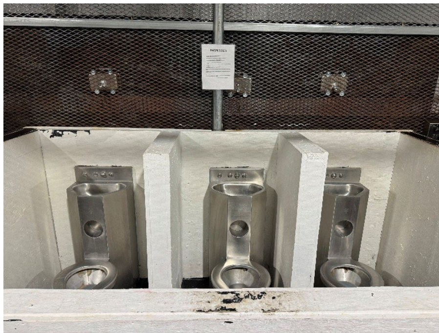
Figure 5. Detainee Housing Unit Toilet and Washbasin Facilities; Observed January 21, 2026
