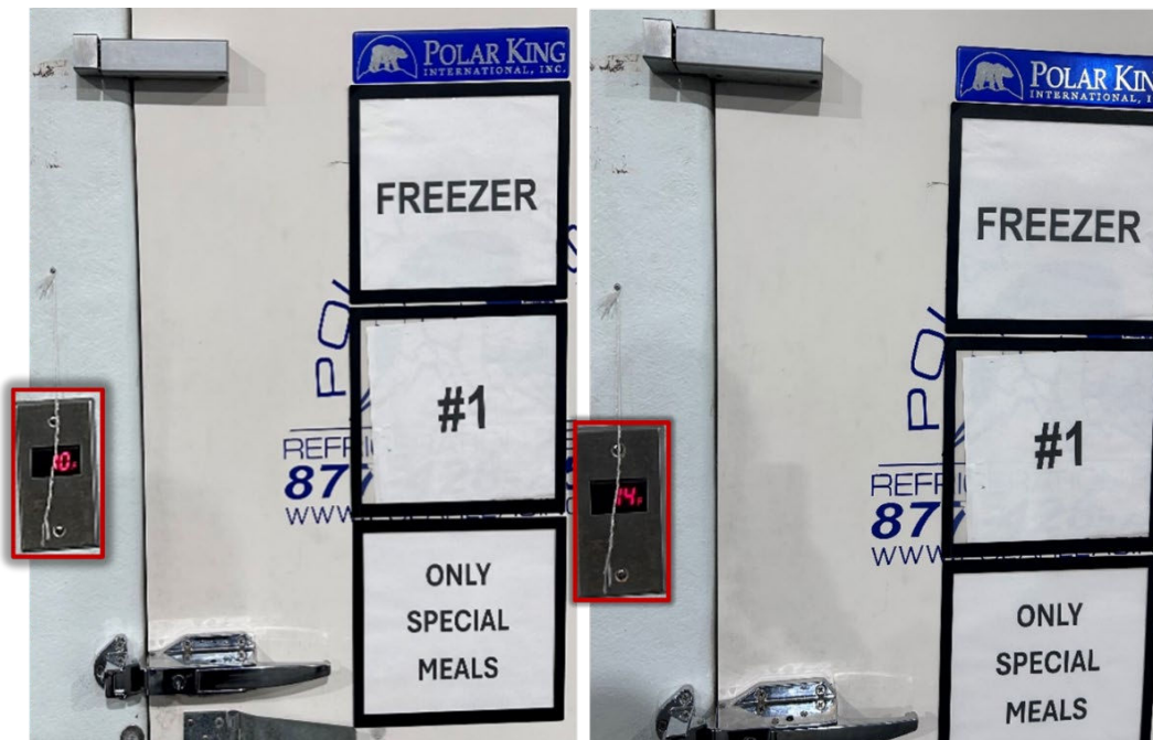
Figures 14 and 15. Freezer No. 1 Exceeding Required Temperature; Observed January 21, 2026
